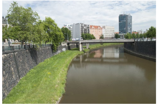
Fig. 114 Narrow, inaccessible berms
